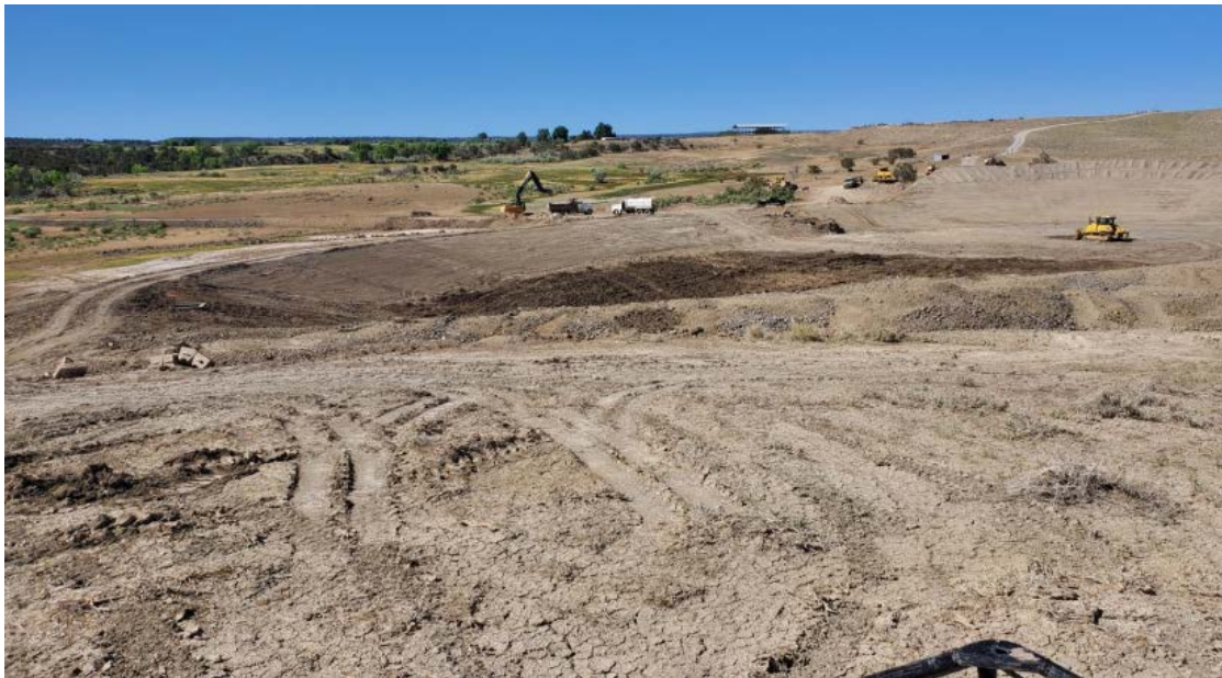
Figure 5 – The 4C regulating reservoir during construction, part of the Crawford Clipper Ditch Company, near Crawford, Colorado
