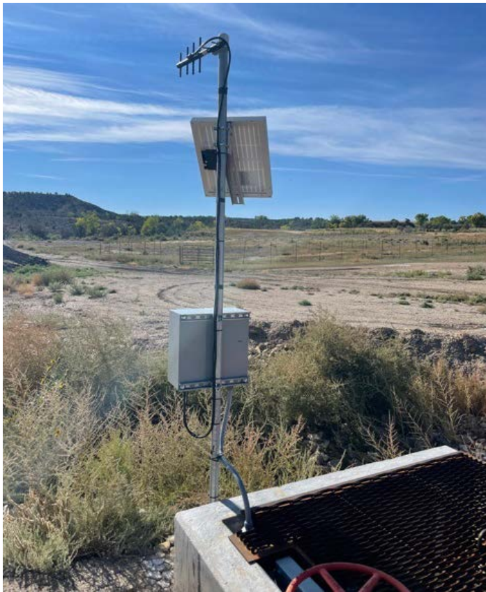
Figure 7 – Solar powered implemented SCADA system component at 4C regulating reservoir outflow, Crawford
