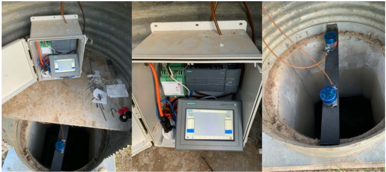
Figure 10 – Implemented SCADA equipment at the Crawford Reservoir Feeder Canal, Crawford, Colorado
