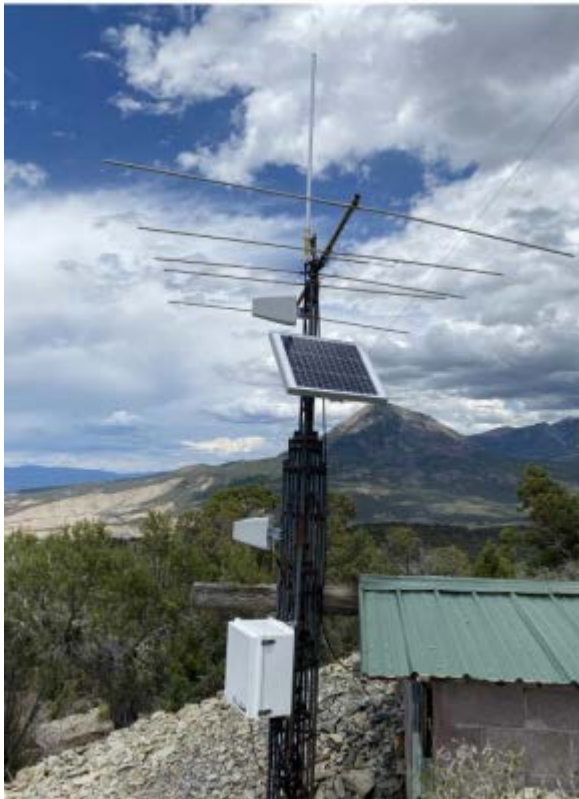
Figure 8 - Young's Peak Communication Station, Crawford, Colorado
