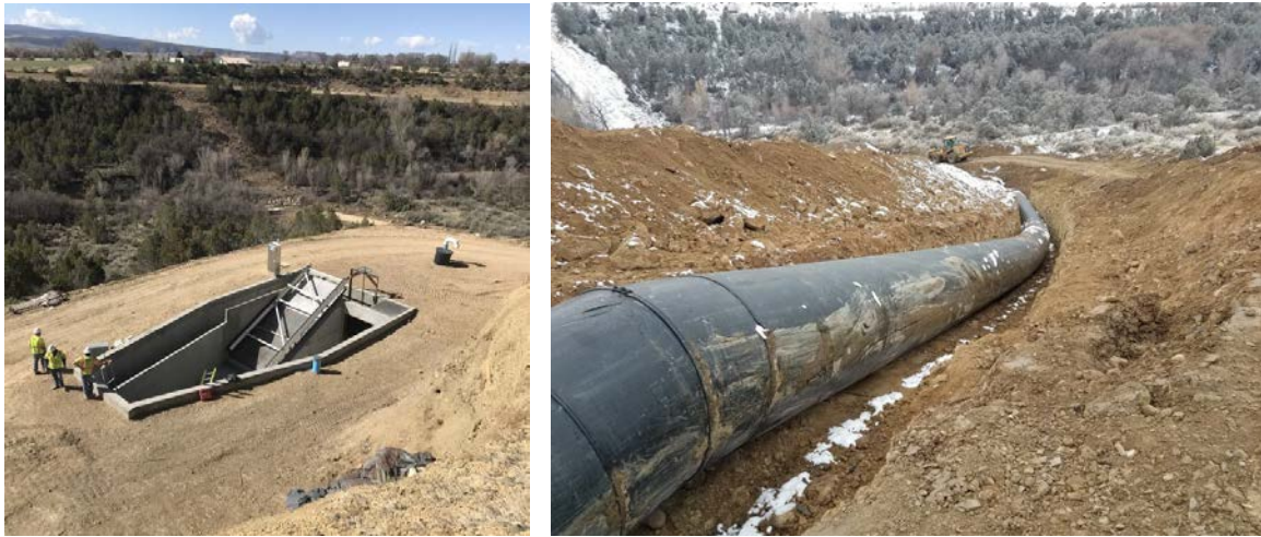
Figure 2 – Fire Mountain Canal Improvement Project: New siphon entrance and screen structure (left) with HDPE piping related to segment 47 pipeline (right)
