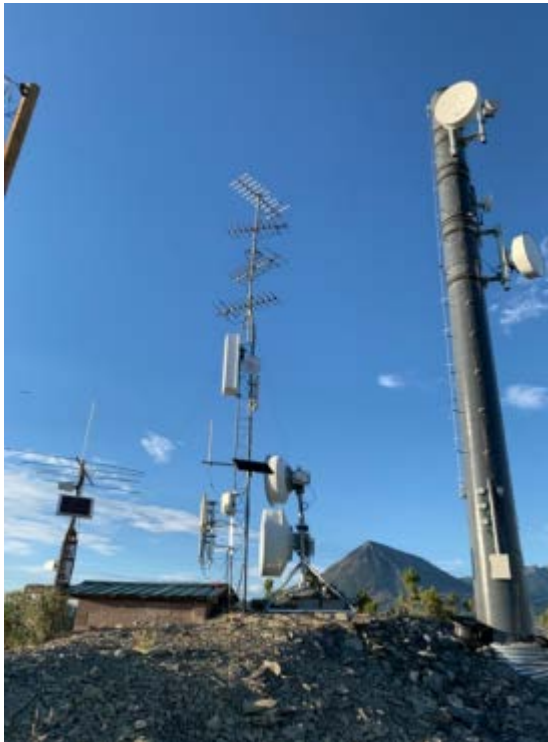
Figure 11 – SCADA network telemetry equipment installed on Young’s Peak tower to assist with the transmission of regional information collected, Crawford, Colorado
